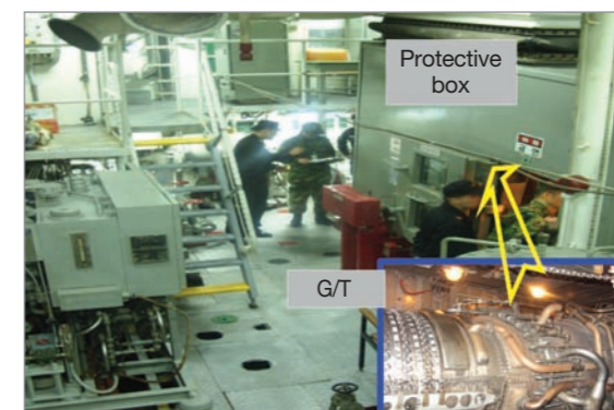
〈Figure II-2-9〉 Gas turbine protective box
