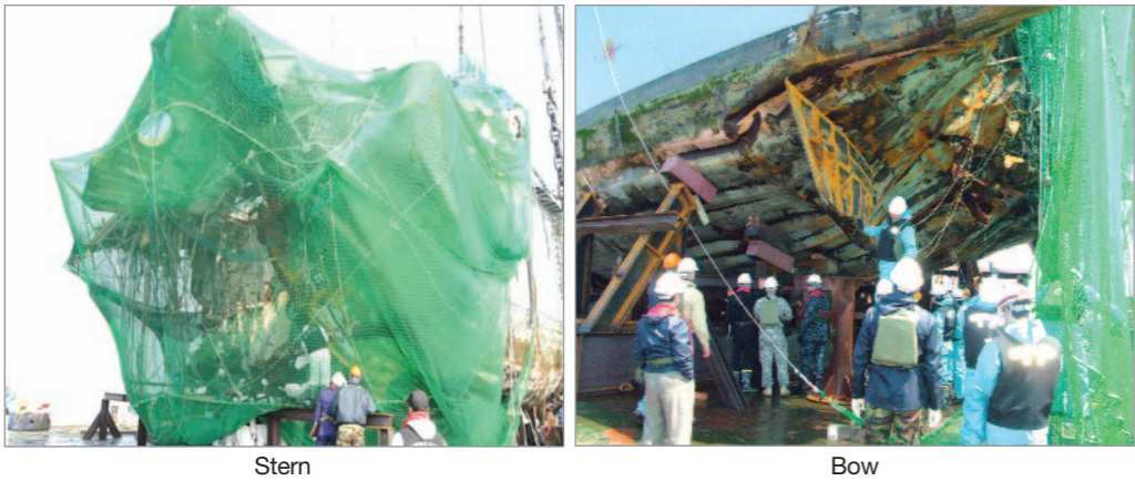
〈Figure III-2-2〉 Collection activities on the barge when the hull was salvaged
